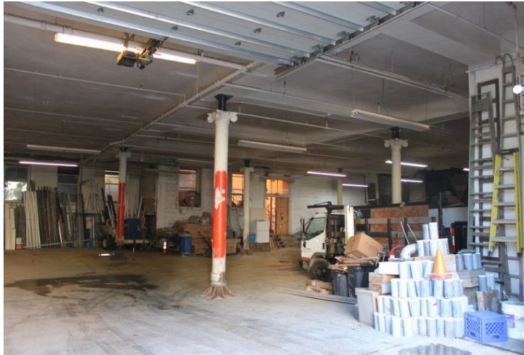
FIGURE 13. CHURCH: BASEMENT SHOWING GUTTED CONDITION, 2015.
