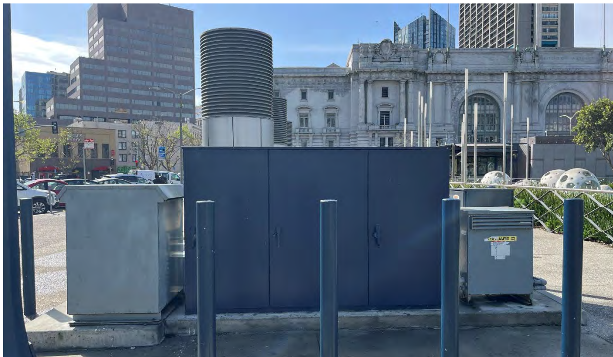
Figure 2. Example Aboveground Cabinet
